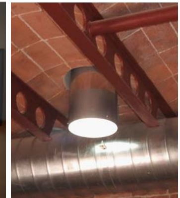
(B) HANGING DIFFUSER (TAILOR MADE!) curved and sloped ceiling
